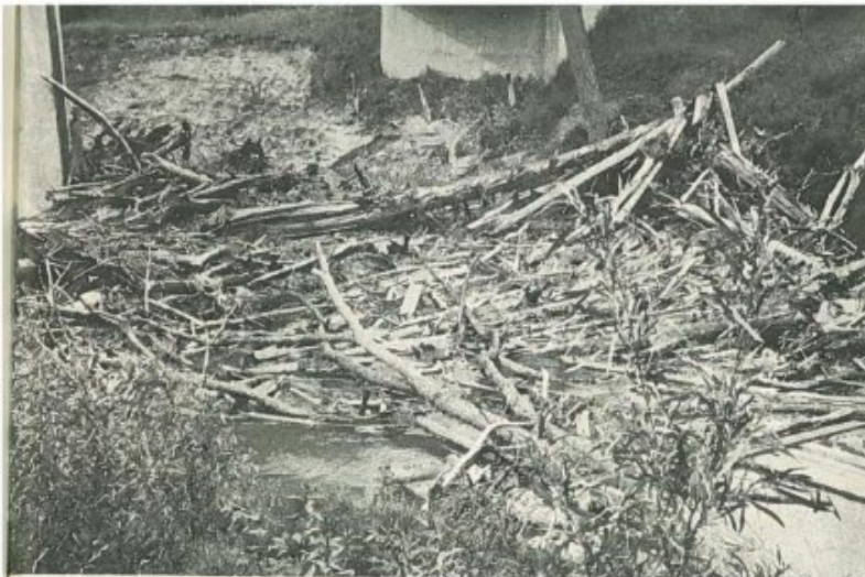
Severe streambank erosion at Nottawasaga River Bridge has resulted from this log jam.
