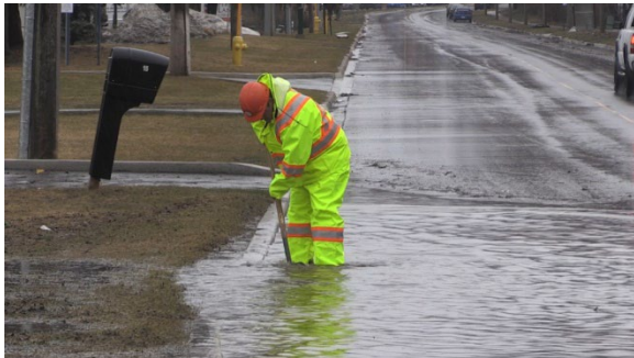
City of Barrie crews work to unclog drains amid heavy rainfall on Wed., April 5, 2023. (CTV News/Rob Cooper)
