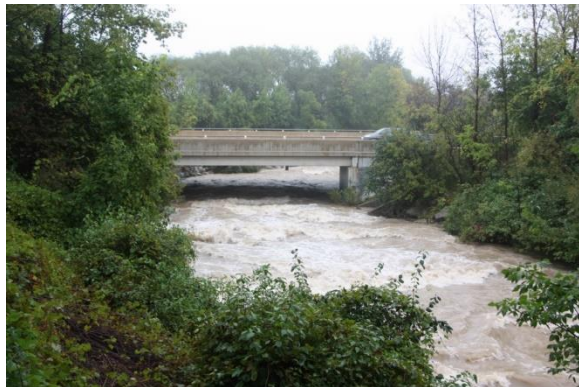
The Pretty River Dike is a two-kilometre structure with a bedrock bottom and steep banks lined with 12- to 18-inch stones. Erika Engel/CollingwoodToday
