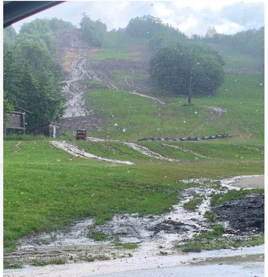
Silt fence does little good
