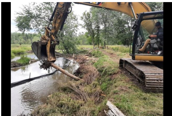
2 / 6 An excavator installs log jams into the river bank to stabilize the soil. Photo supplied by the Nottawasaga Valley Conservation Authority
