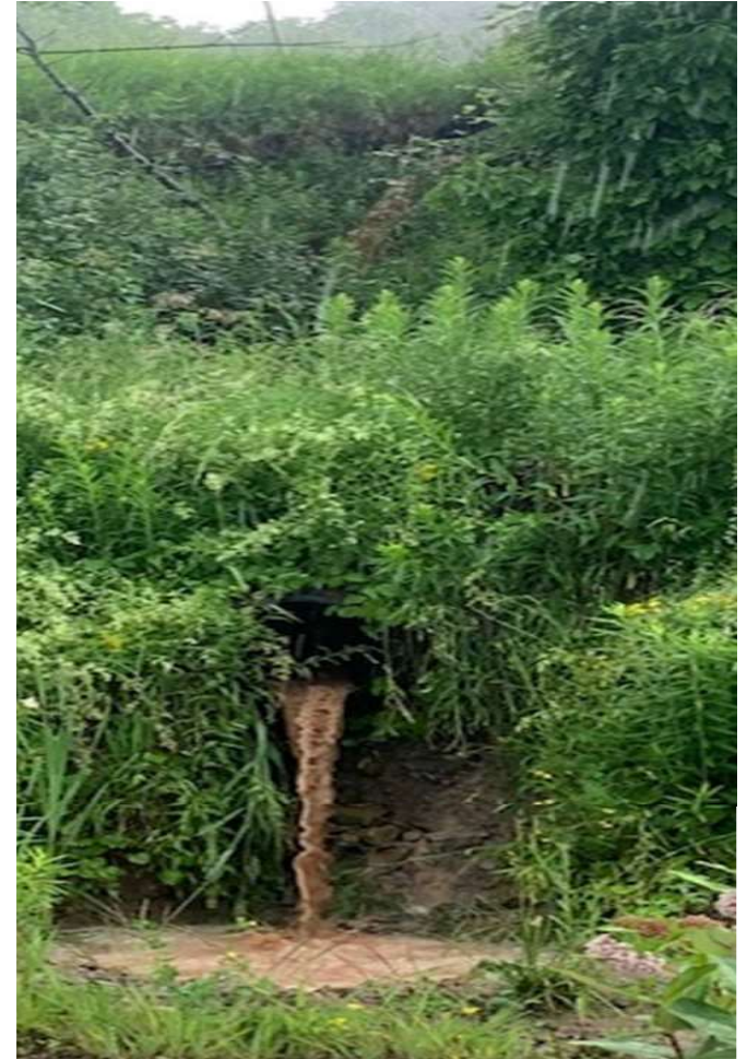
Watercourse 10 – June 26 2023 North Lot at Craigleith Ski Club - Not just a spring occurrence
