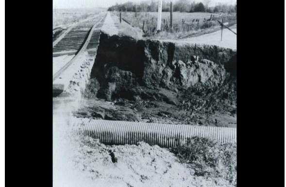
3 / 7 Hurricane Hazel washed out this road in 1954.Photo supplied by the Nottawasaga Valley Conservation Authority
